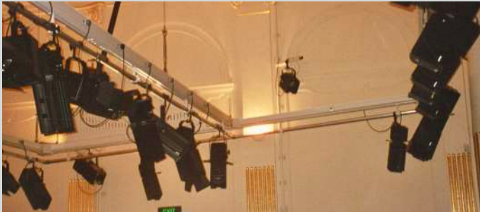
New lighting grid.
